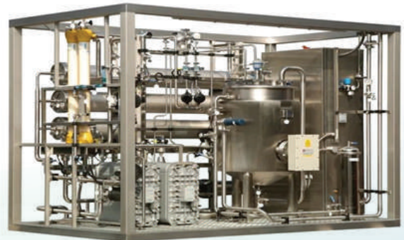
Purified Water Generation Plant
